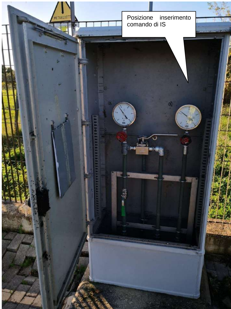
Foto 15 – armadio isolation system
